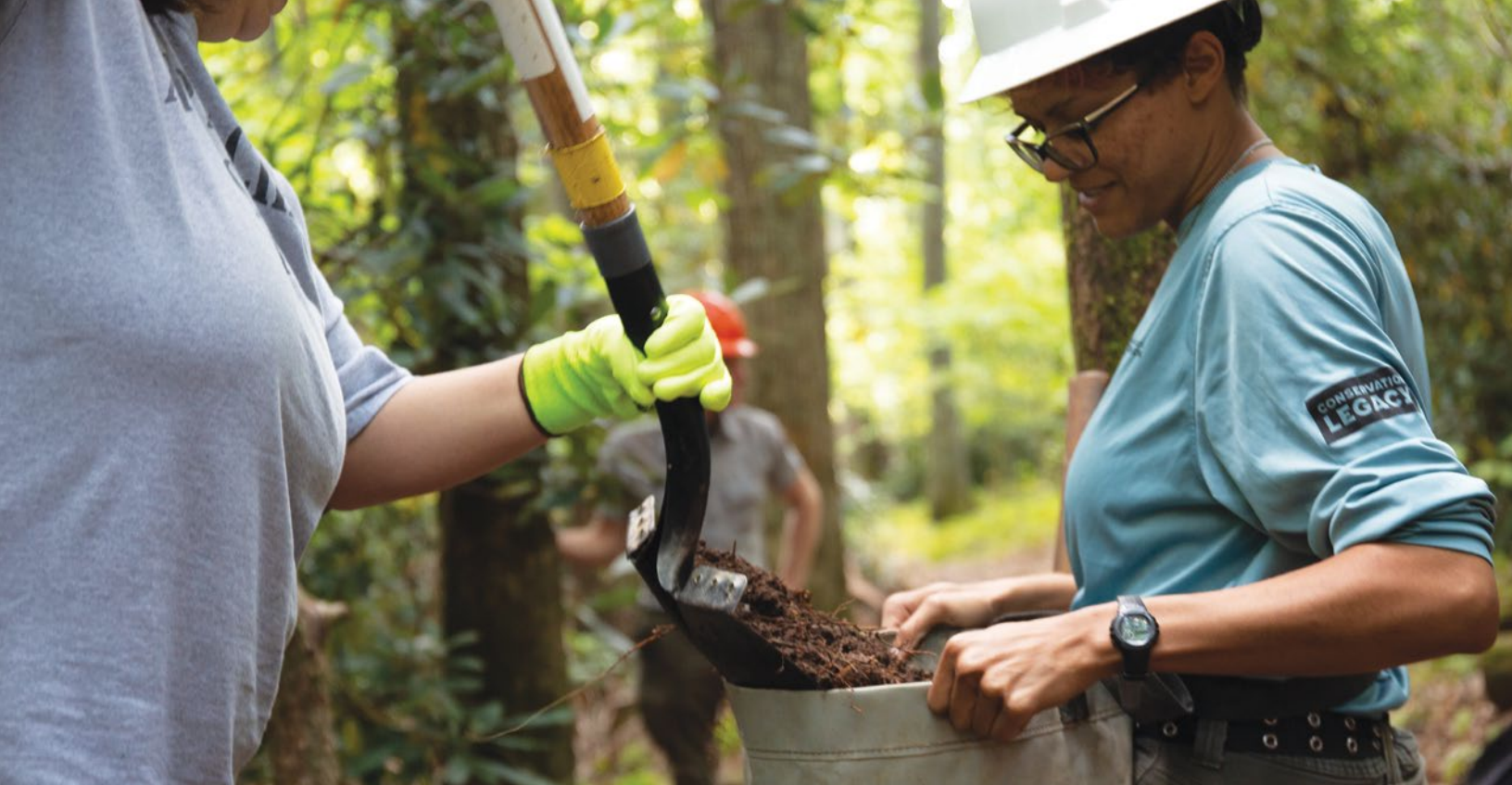
Crew member Tiara Atkins at the site of repair work on the Tanawha Trail. Photo by Torri Pelletier/Conservation Legacy
