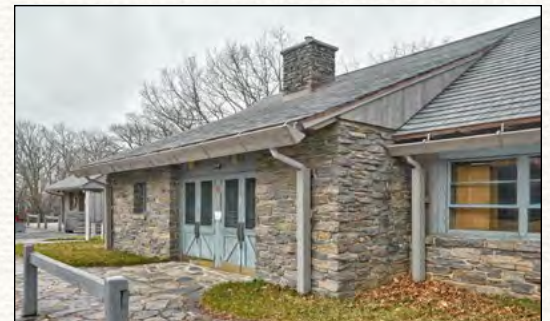
A new roof is one of the many repairs your donations have made possible at The Bluffs.
