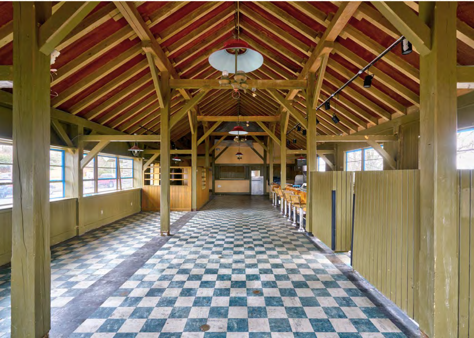
In March, renovation began on The Bluffs Restaurant's interior in preparation for its reopening this summer. Photos by David Huff
